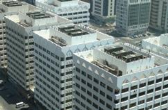
Roof Top Chillers
